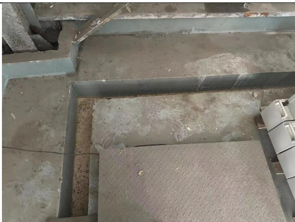
△144m 2 危废仓库导流渠
