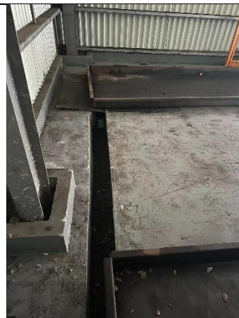
△144m 2 危废仓库泄漏液收集池
